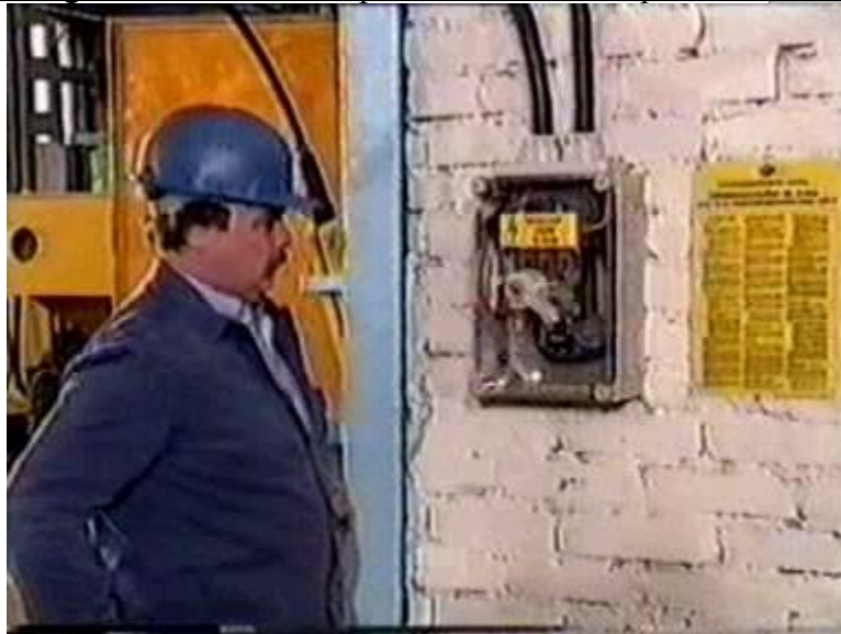
Accesul la tabloul electric general
